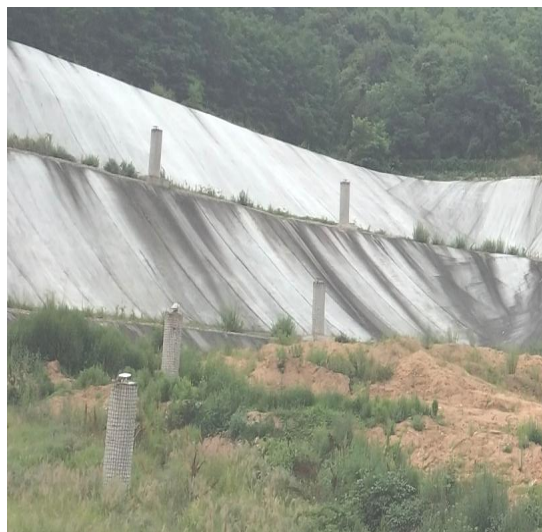
填埋区导排井
